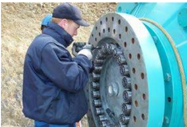
Flange coupling of the gear box on a wind turbine. An expansion bolt with integrated Superbolt technology is used to transmit the enormous torque. The solution is also compact and does not add a lot of weight, which was a requirement.
