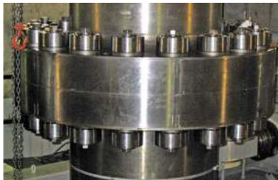
Superbolt expansion bolts are ideally suited for shaft couplings, as seen here on this Francis type pump/generator shaft coupling at a pumped-storage facility.
